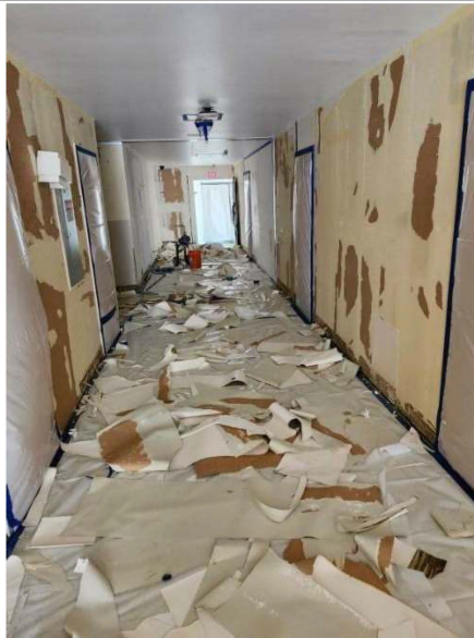
Due to leaks in multiple locations, water was detected within the walls and electrical panels in the hallway leading to and inside the Standby Emergency Department. Abatement was required.
