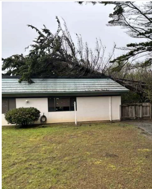
In the image above, a large tree fell onto the roof in the area where the Standby Emergency Department is located and punctured parts of the roof, causing structural damage and significant leaks into the building.
