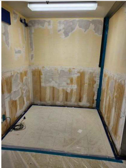
The above image shows walls being removed in the Standby Emergency Department for abatement throughout the Department and within its walls.
