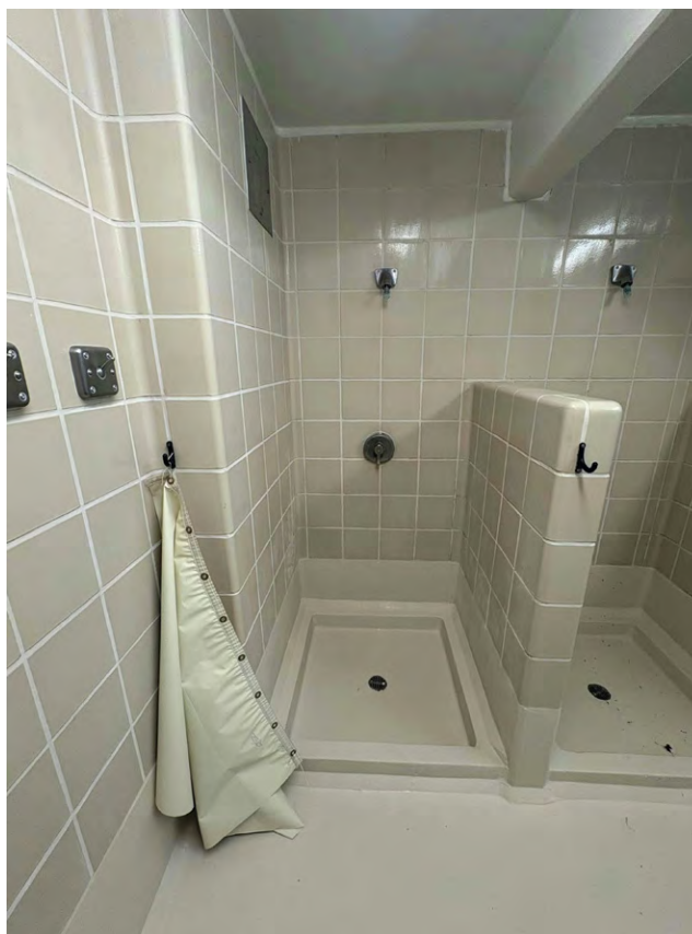
Figure 62. Shower Facilities at Cal City
