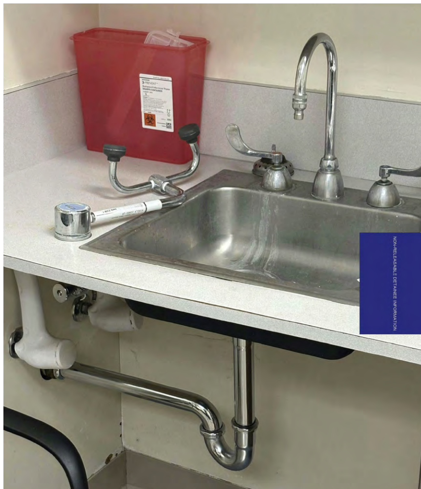
Figure 67. Sink in Medical Area at Cal City
