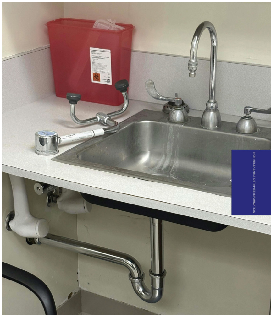
Figure 67. Sink in Medical Area at Cal City
