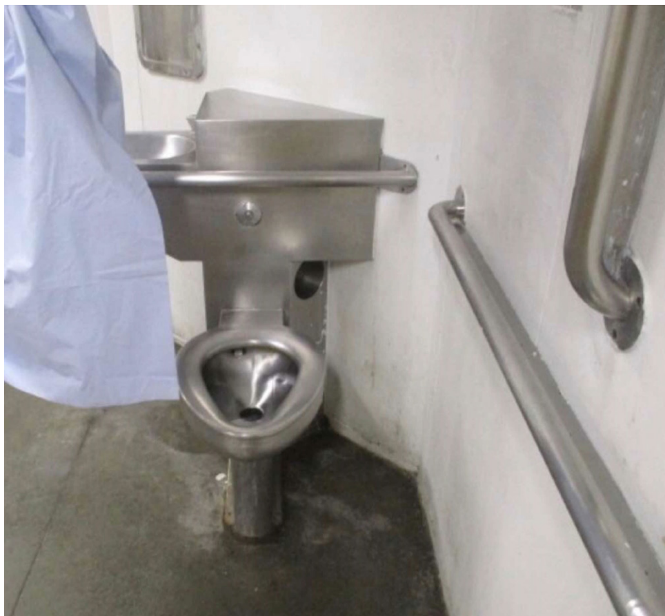
Figure 45. Intake Holding Cell Toilet with Sink at Otay Mesa
