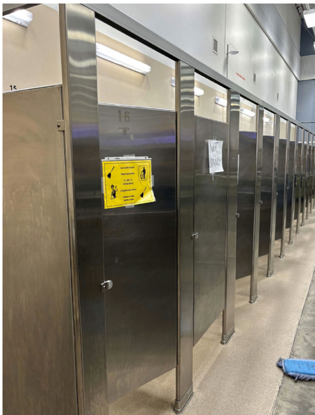
Figure 51. Doors to Toilet in Housing Unit at Otay Mesa
