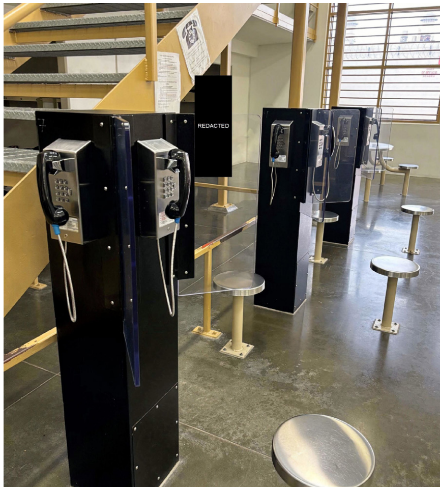
Figure 53. Telephones in Housing Unit at Otay Mesa
