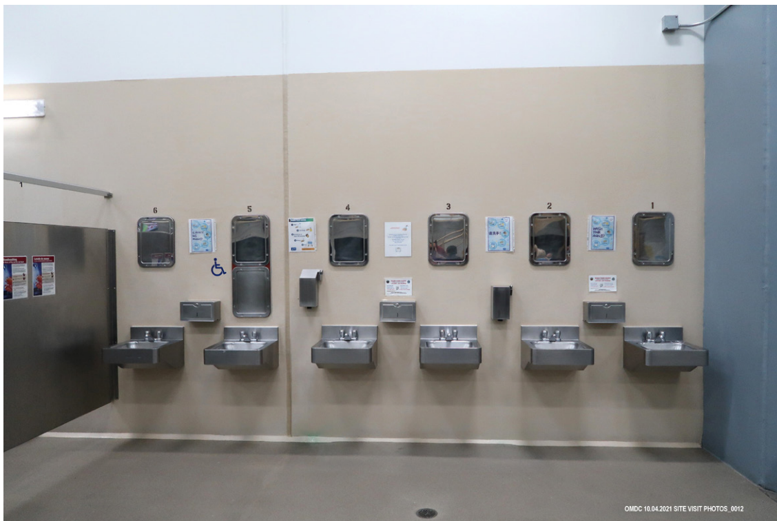
Figure 50. Sinks in Housing Unit at Otay Mesa
