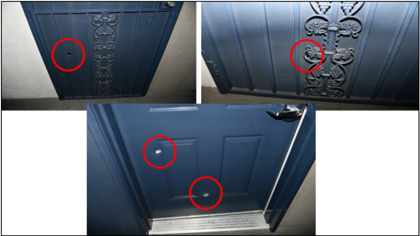
Strike marks on screen door and interior door
