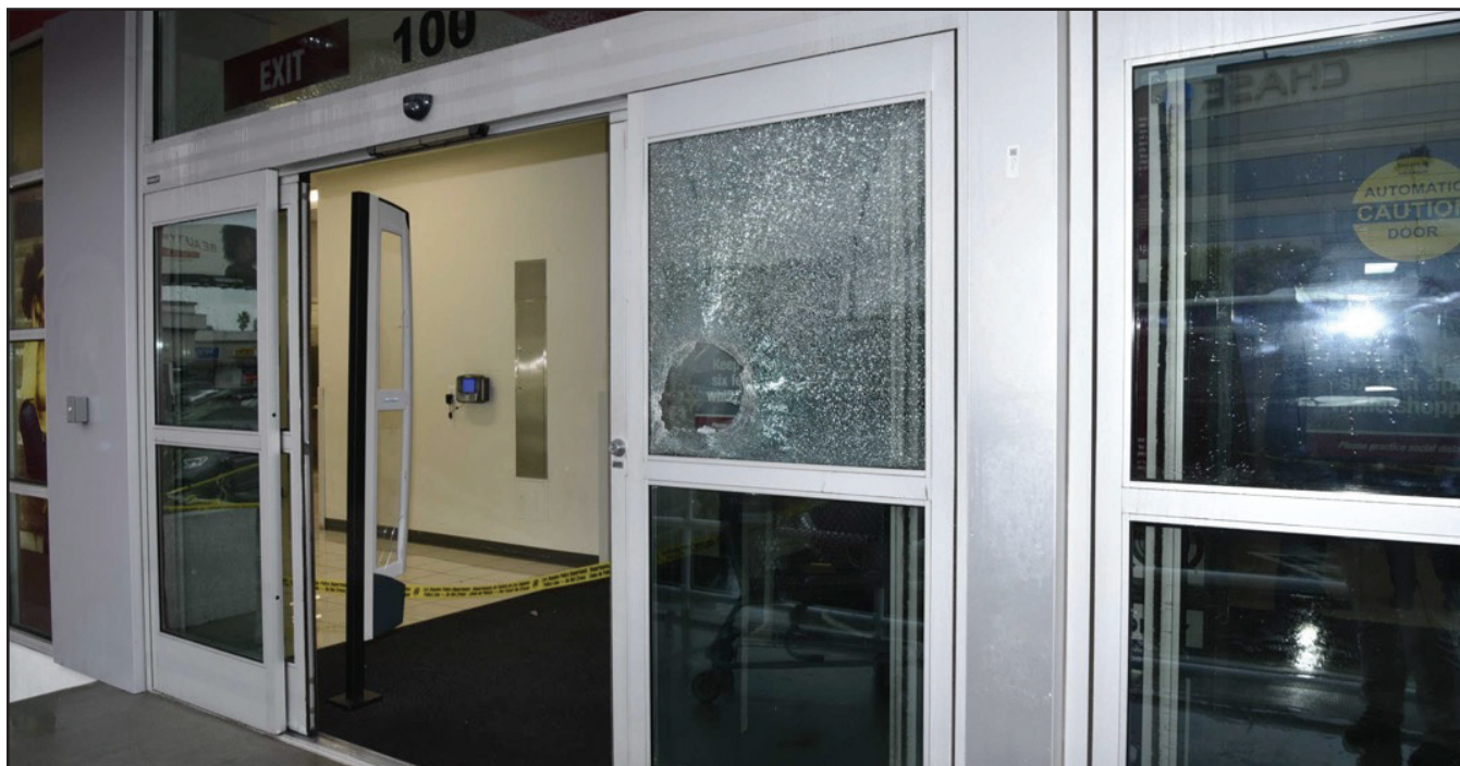
The broken glass panel in Burlington's front door
